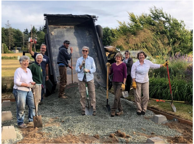
Laying the foundation for the greenhouse. Left to right: Carole Matthews, Barb Douglas, Ken Hess, Delivery staff, Ilze Zigurs, Barb Schmitt, ??, Tristy Nielsen
